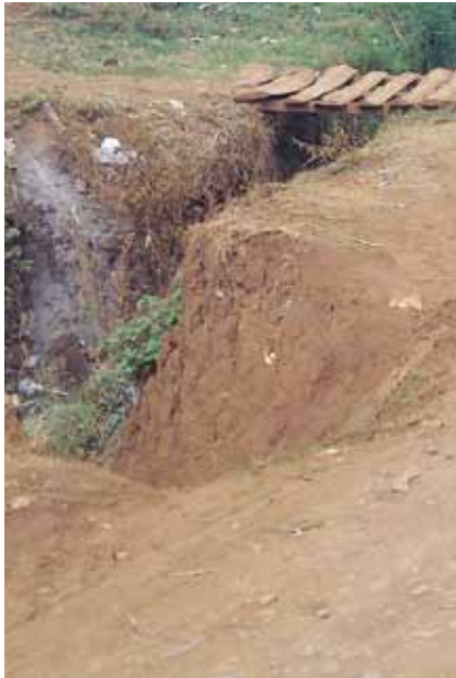
Fig. 2.5. Eroding sidedrain, Mutomo town
