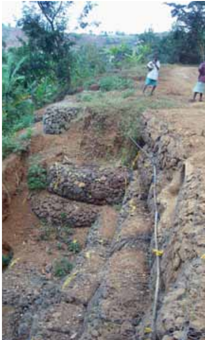
Fig. 2.16. Undersized culvert, Mikinduri-Miathene Road
