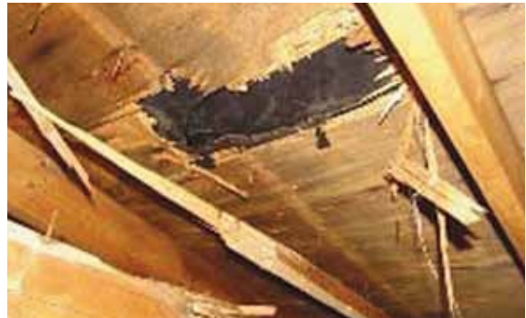
Fig. 4.3. Indoor residential damage from ground vibrations
