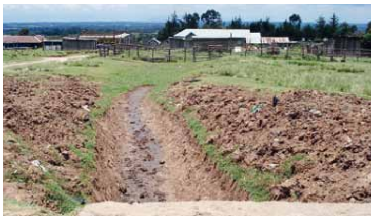
Fig. 2.4. Poorly designed road drainage onto farmland
