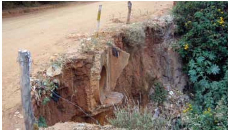
Fig 2.7. Inadequate drainage system, Miathene
